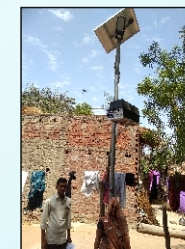
500 PV Street Lighting Systems were installed in Fatehpur district of Uttar Pradesh
