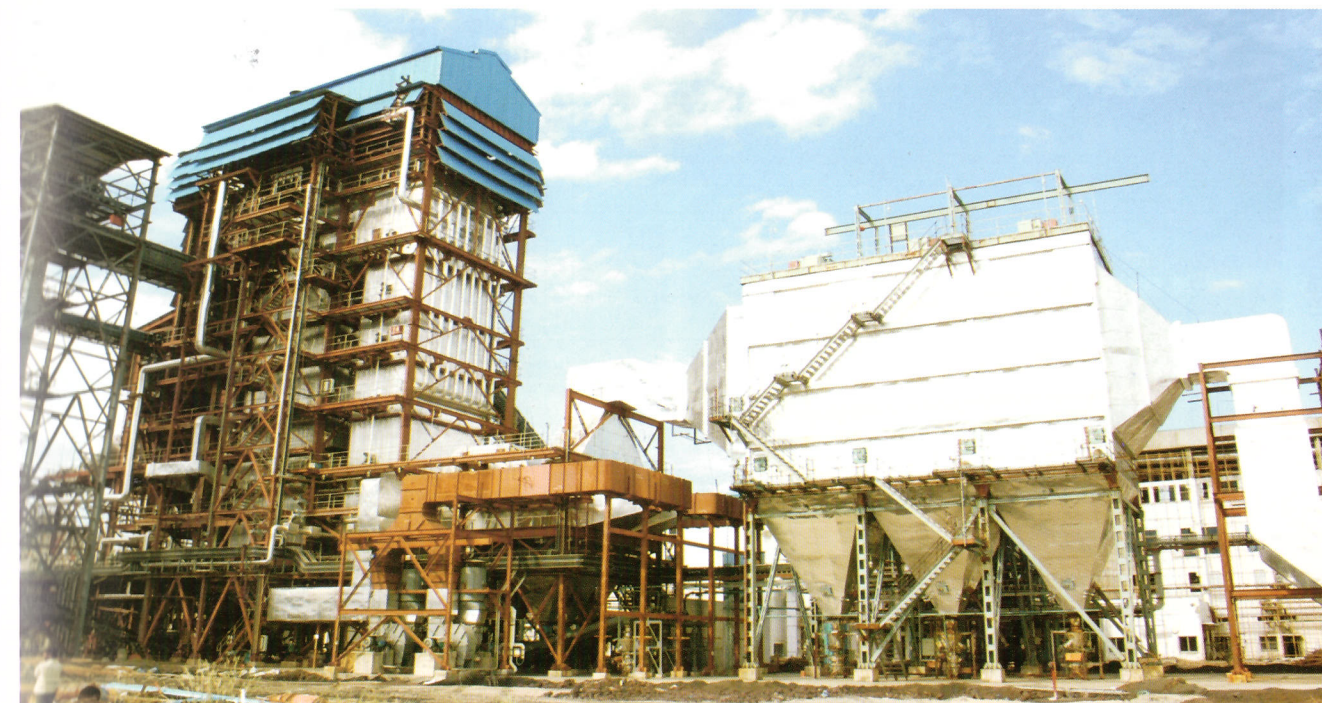
IREDA funded 23 MW Bagasse based Cogeneration project at Udambiyar, Veppanthathi Taluk, Perambatur District, Tamilnadu
