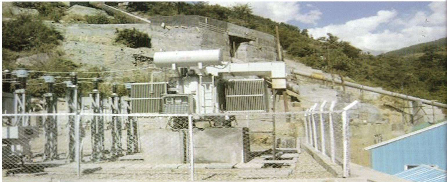
View of Switchyard IREDA funded 5 MW Upper Taraila SHP Project at Chamba Distt., Himachal Pradesh
