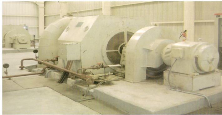
Wide View of Power House Showing Turbines and Generator
