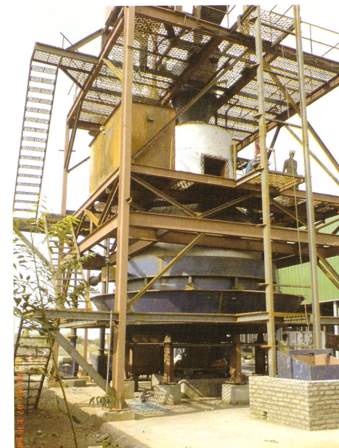
View of Gasifier Reactor of 6 MW th Gasifier
