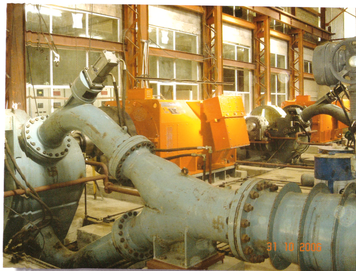
Inside view of IREDA financed 3 MW Lodhama Small Hydro Project set up in Darjeeling District, West Bengal
