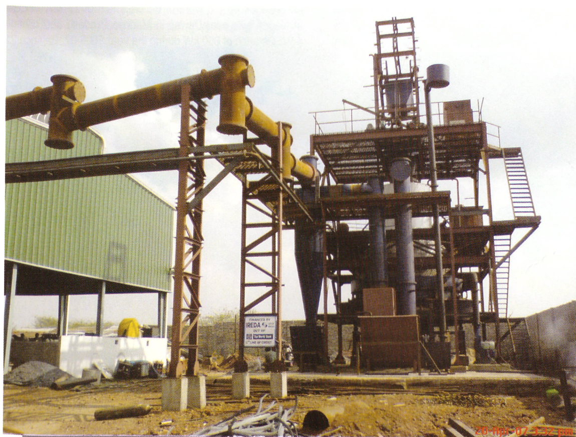
IREDA financed 6 MW th Gasifier for Thermal Application Project at Village Aswathapuram, Kurnool, Andhra Pradesh.
