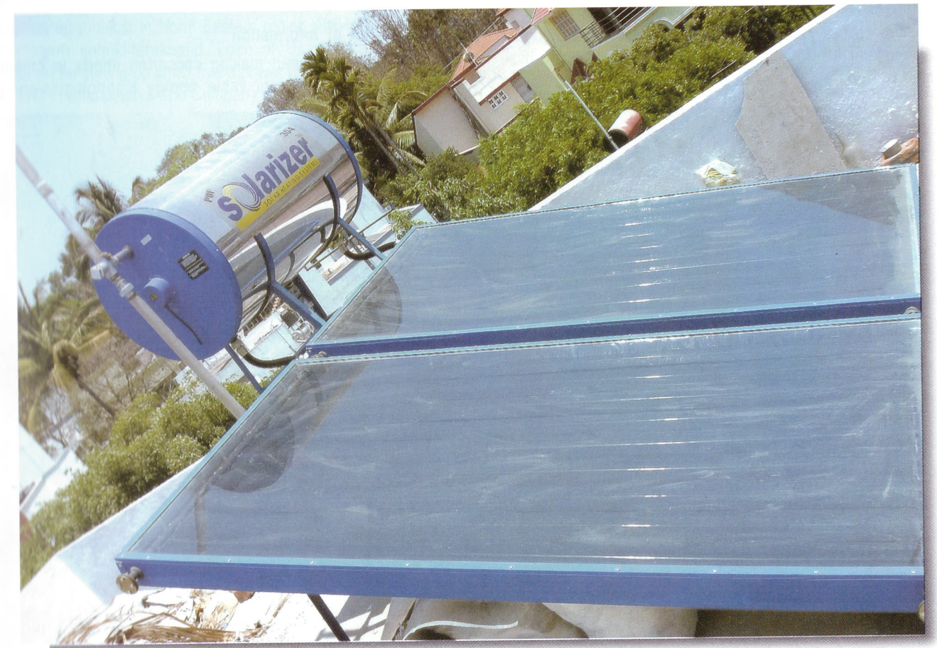
IREDA financed Solar Water Heating System under MNRE Interest Subsidy Scheme
