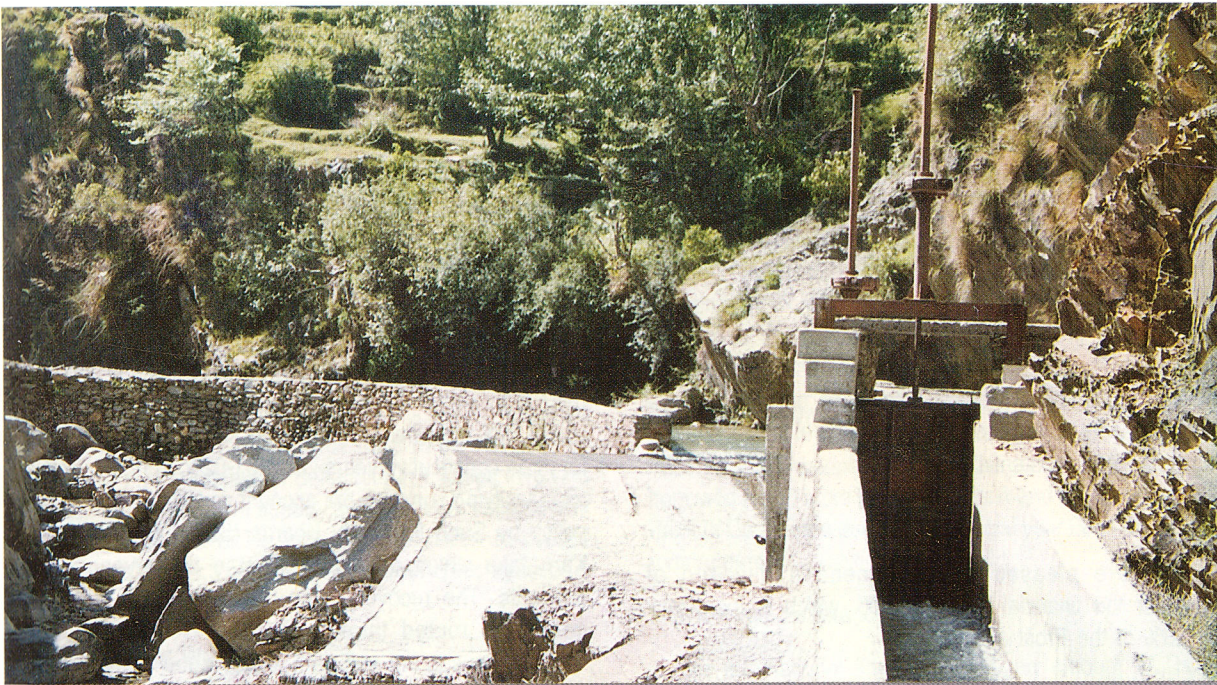
A view of diversion weir with regulation gate of Small Hydro Project set up at Chamba District, Himachal Pradesh with IREDA's assistance.
