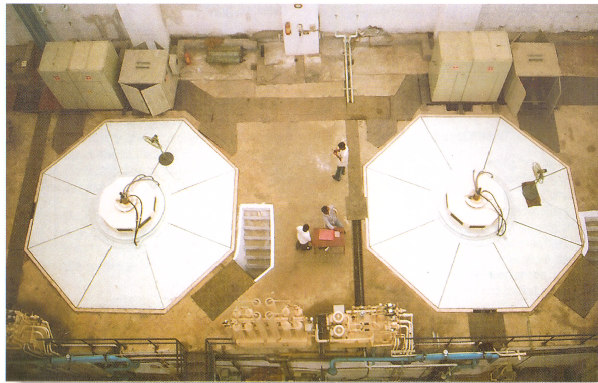
IREDA financed 10 MW Small Hydro Project set up at Nellore District, Andhra Pradesh under World Bank Line of Credit.
