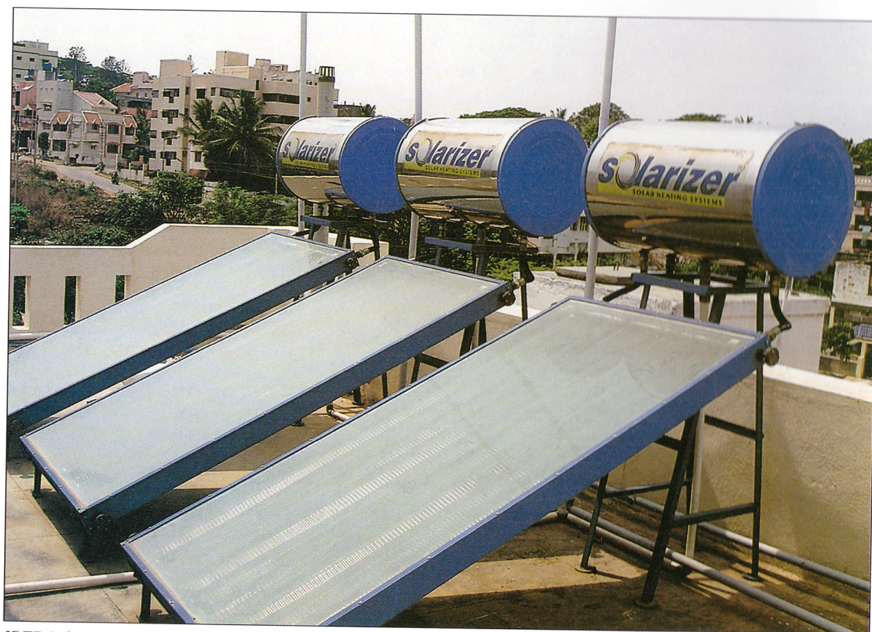
IREDA financed 300 LPD Solar Water Heating Systems installed at roof top of a hotel in Bangalore, Karnataka under Intermediary category.
