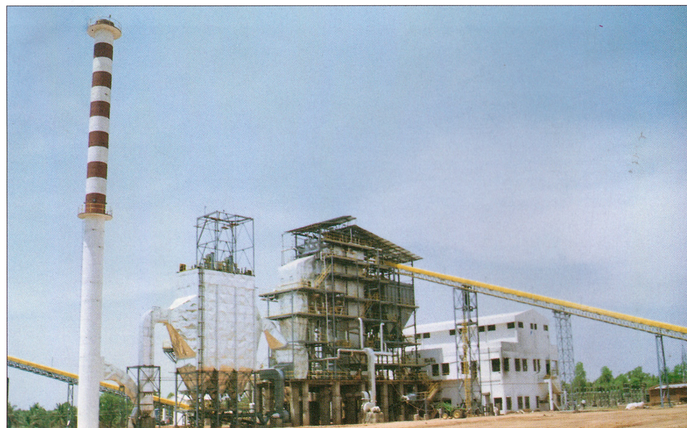
IREDA financed 6 MW Biomass Power Project under implementation in Tumkur District, Karnataka.
