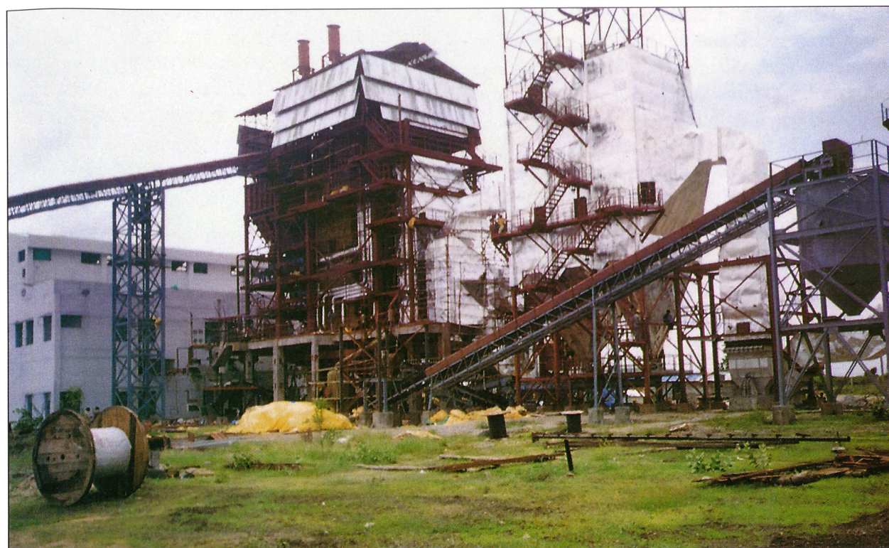
IREDA financed 6 MW Biomass Power project being setup in Raichur District, Karnataka.
