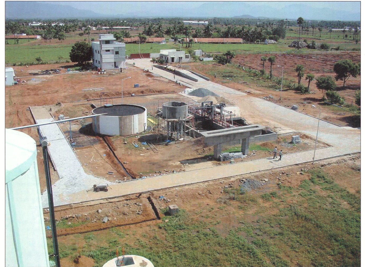
IREDA financed 1.50 MW Poultry Waste to Energy Project being set up at Namakkal District, Tamilnadu.
