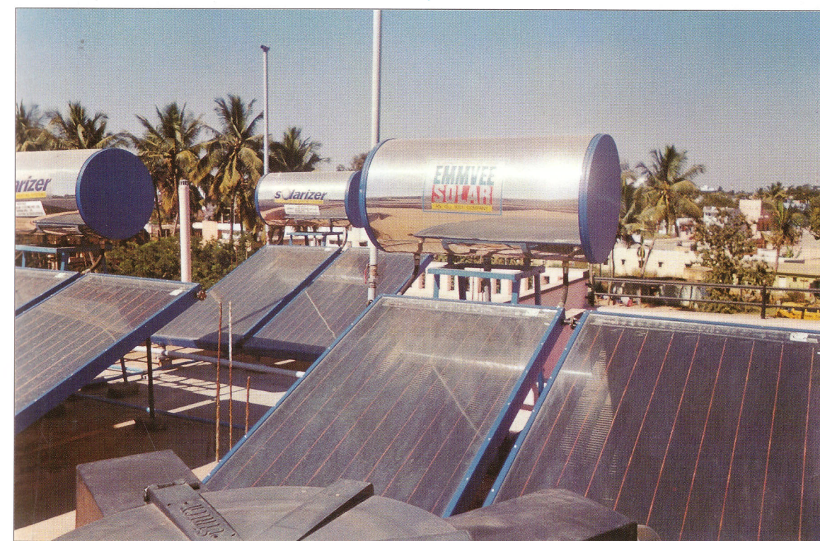
600 LPD Solar Water Heating systems installed at Bangalore, Karnataka under direct users category with IREDA's assistance.
