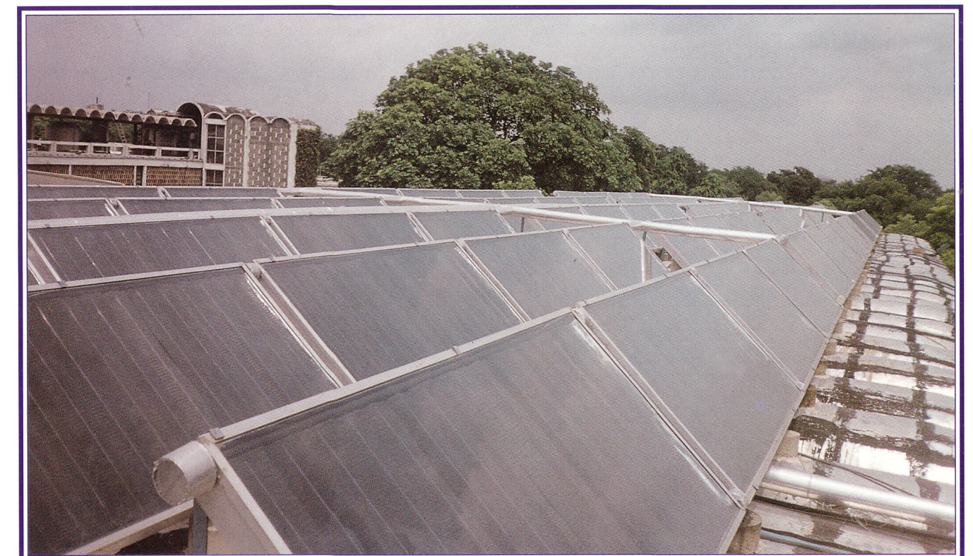
11000 LPD Solar Water Heating System for Canteen application installed at New Delhi under direct user category with IREDA's assistance.
