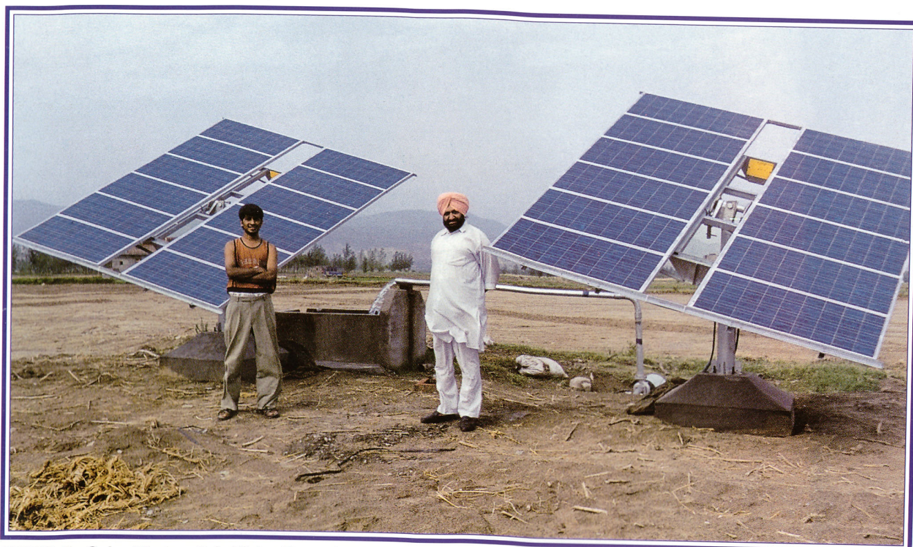
1800 Watts Solar Photovoltaic Water Pump installed under MNES Programme through IREDA at Punchkula, Haryana.
