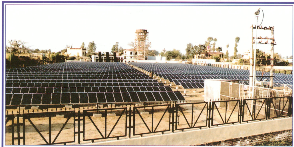
IREDA financed 200 kW Solar Photovoltaic Power project set up with IREDA's financial assistance at Nawanshahar district of Punjab.
