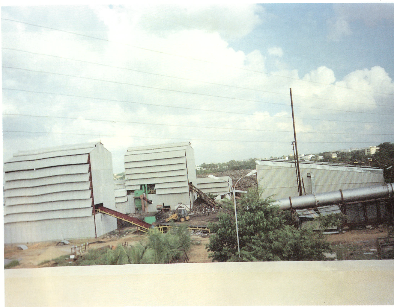
IREDA financed 210 TPD Fuel Processing Plant set up at Gandamguda Village, Ranga Reddy District, Andhra Pradesh.
