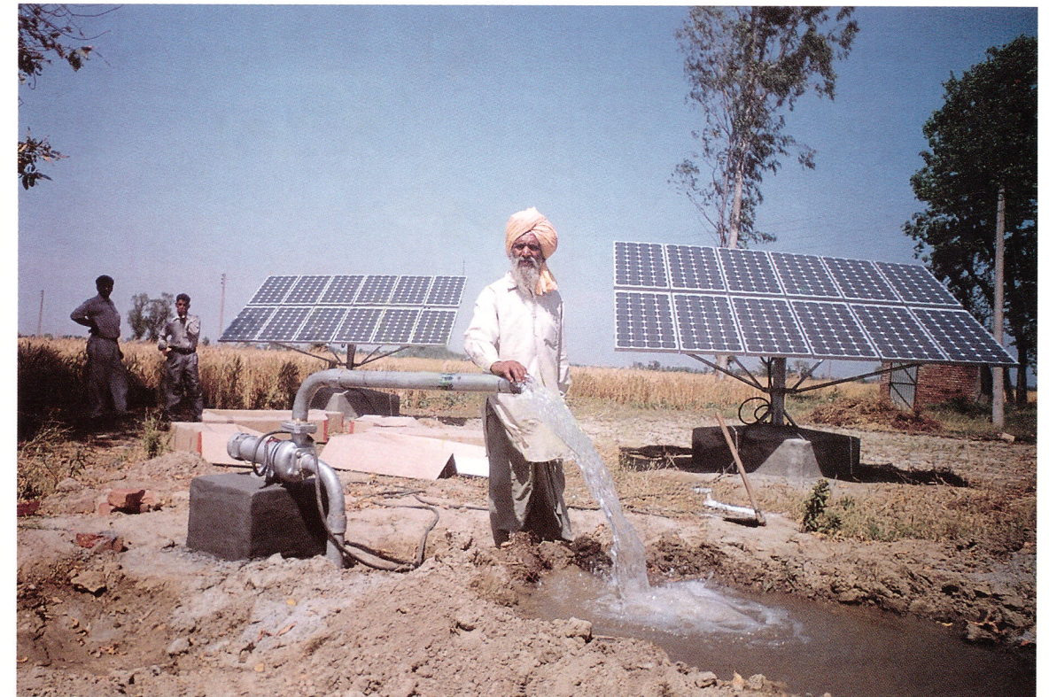
Solar Photovoltaic Water Pump installed under MNES Programme for the year 2001-02 through IREDA at Bhatnora Village, Block Bhogpur, Jalandhar District, Punjab.
