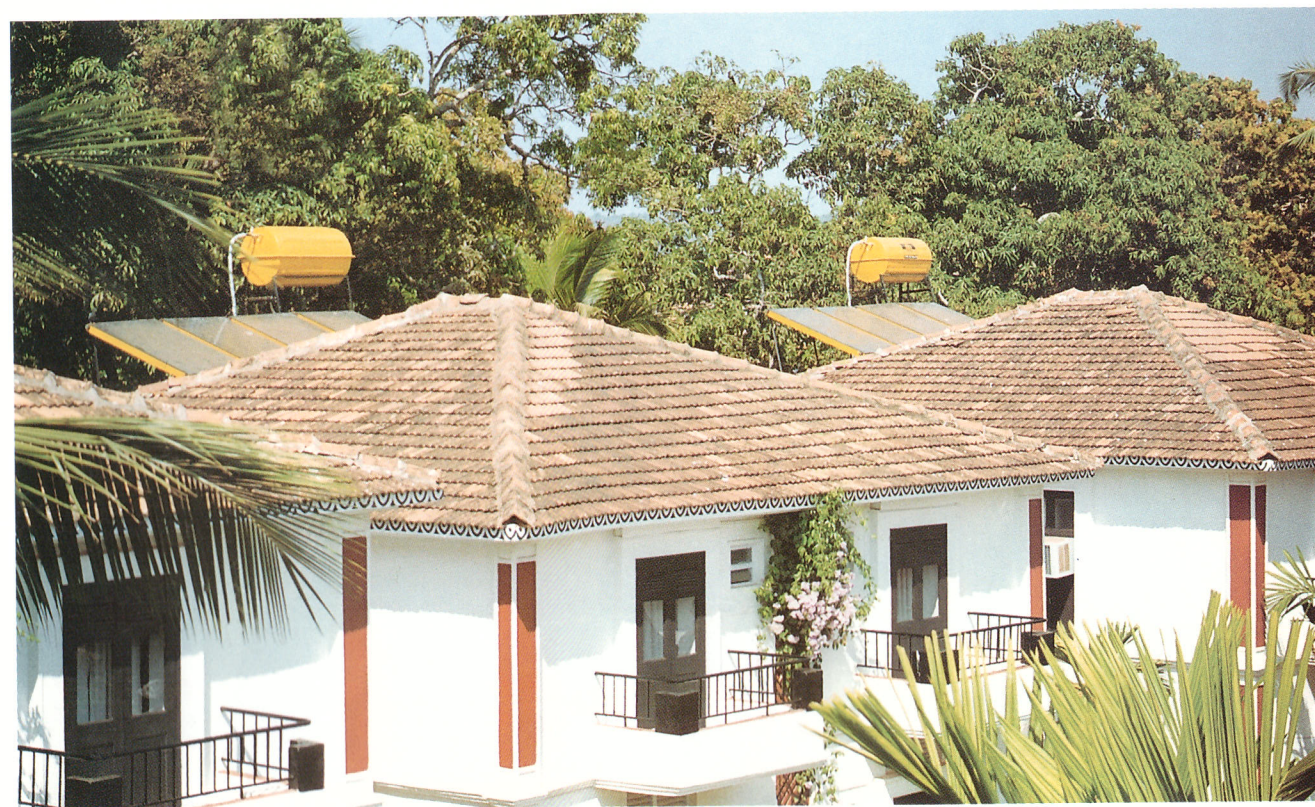
IREDA financed 5400 LPD Solar Water Heating System installed in a Resort in Goa.
