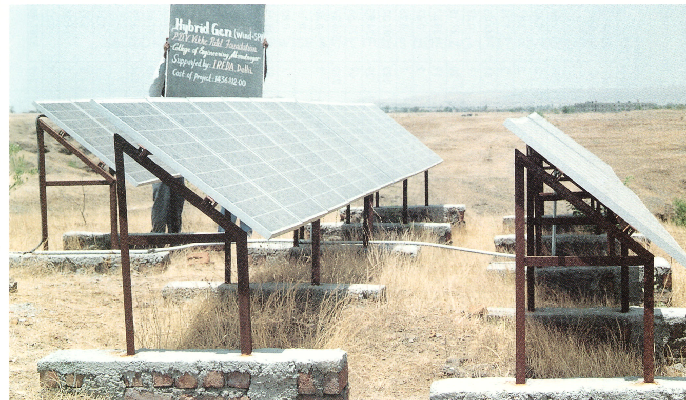
5 KWp capacity Hybrid Solar Photovoltaic Wind Power plant installed in Ahmednagar, Maharashtra under SPV Market Development Programme sanctioned by the World Bank to IREDA.
