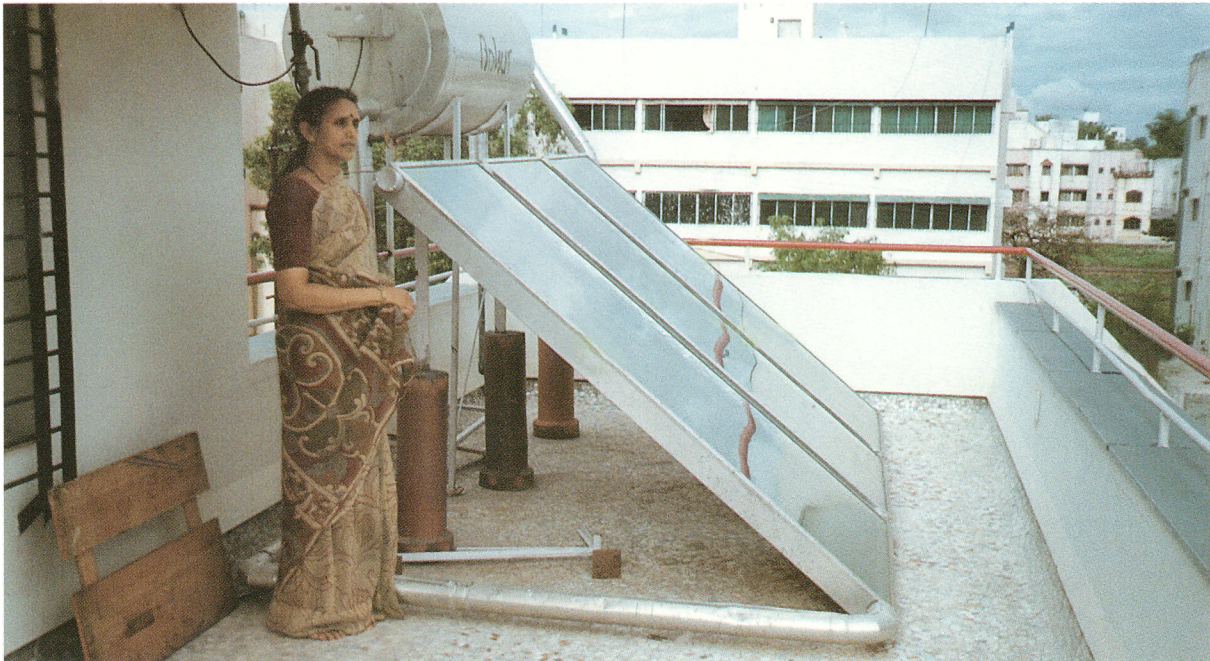
IREDA financed 300 LPD Domestic Solar Water Heating System installed at 'Aakar' Tidalce Colony, Nasik, Maharashtra under intermediary scheme.
