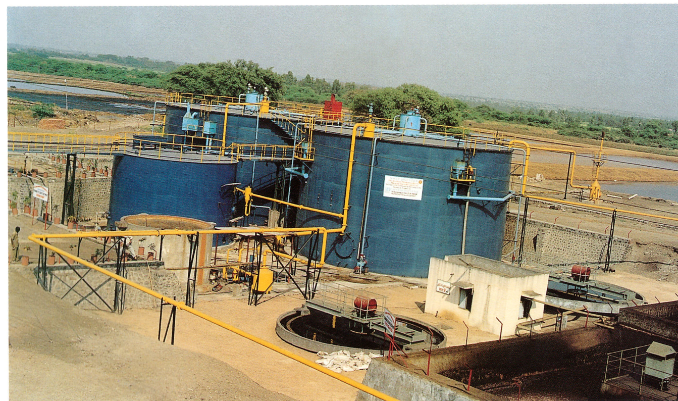
IREDA financed 1 MW Biomethanation industrial effluents Power Project set up at Shreepur, Malshria Tehsil, Solapur District, Maharashtra.
