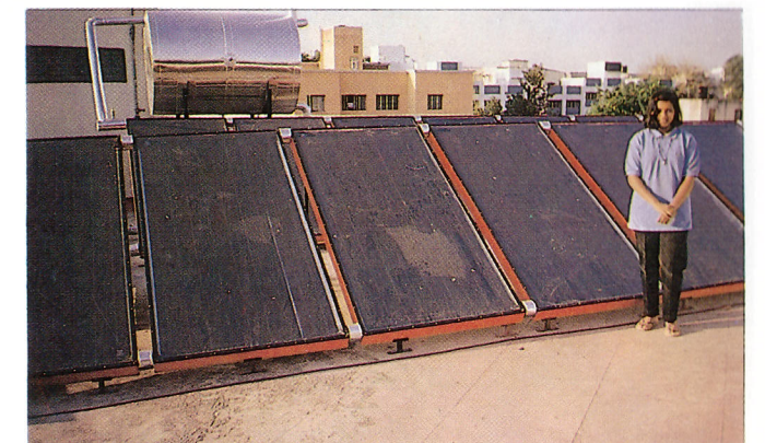
IREDA financed 1000 LPD capacity Solar Water Heating System installed at Ladies Hostel at Pune under Solar Thermal Intermediary Scheme.
