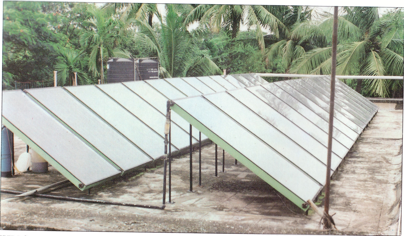
IREDA financed 4000 LPD Capacity Solar Water Heating System installed at a hotel in Mumbai.
