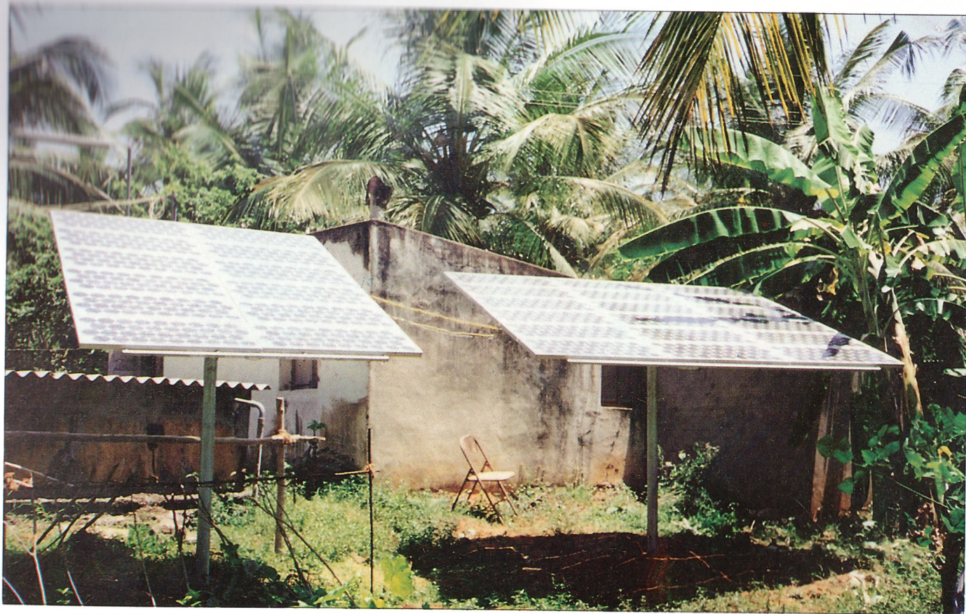
Solar Photovoltaic Water Pump installed under MNES Scheme through IREDA in Karwar district, Karnataka.
