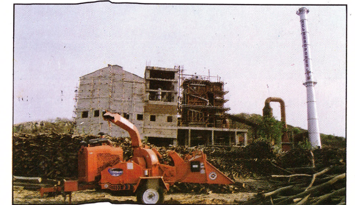
IREDA financed 6.75 MW Biomass Power Project set up at Vedadri village, Krishna district, Andhra Pradesh.
