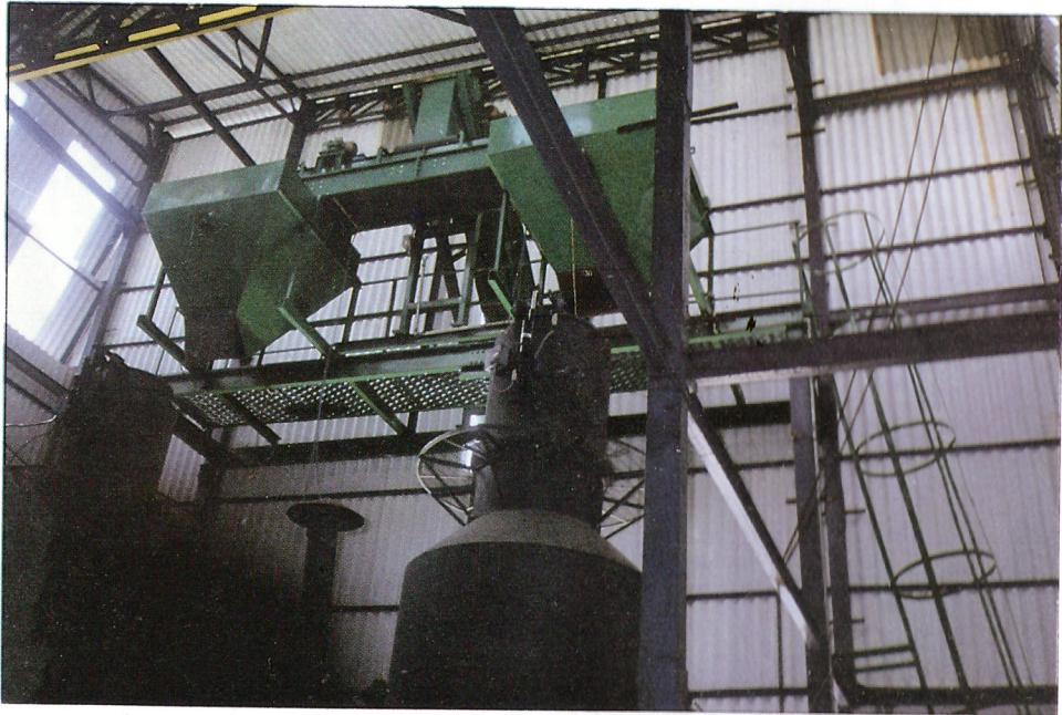
IREDA financed 1 MW Biomass based Gasifier plant setup in Jigani Village, Karnataka
