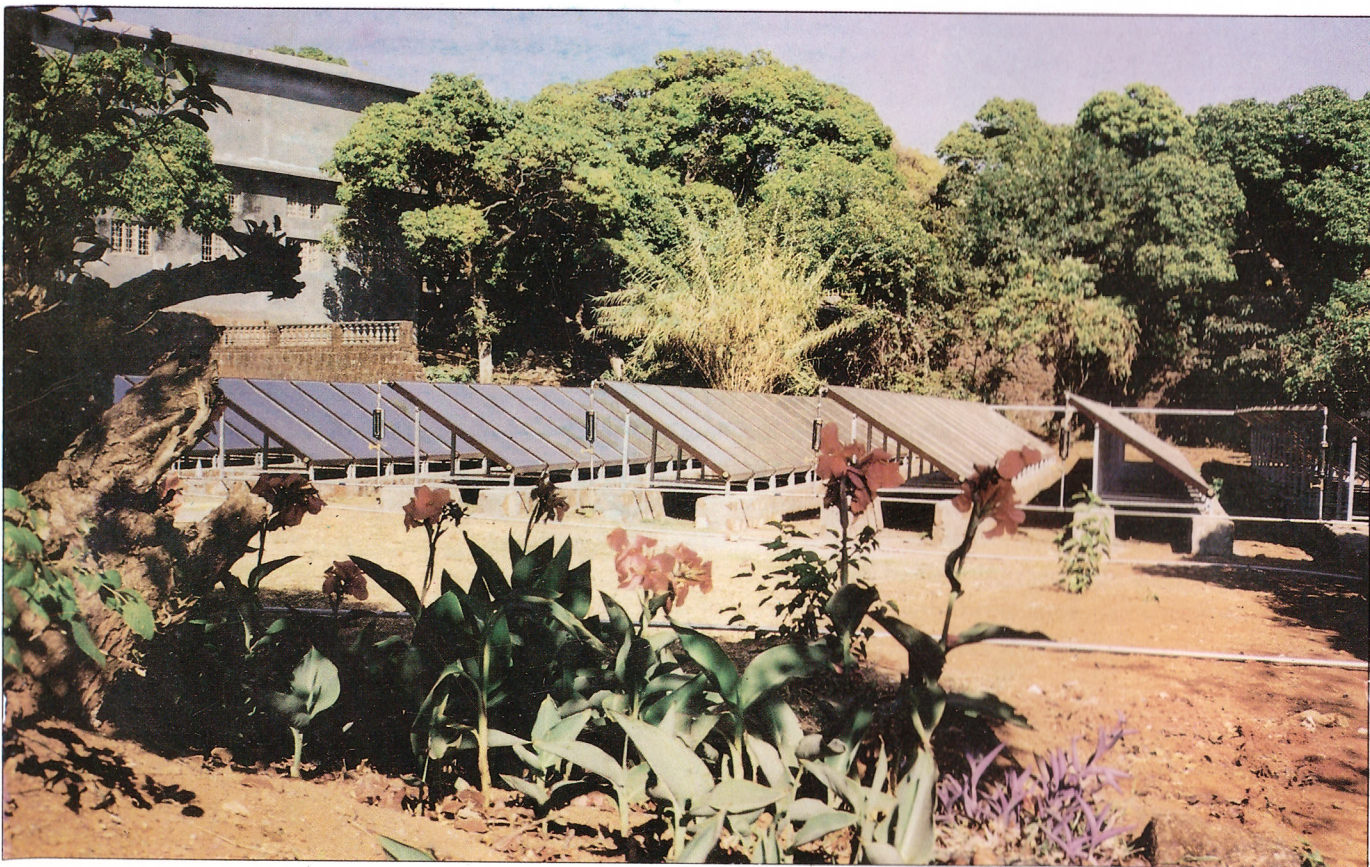
IREDA financed 13000 LPD capacity Solar Water Heating System installed in a Hotel in Mahabaleshwar, Maharashtra
