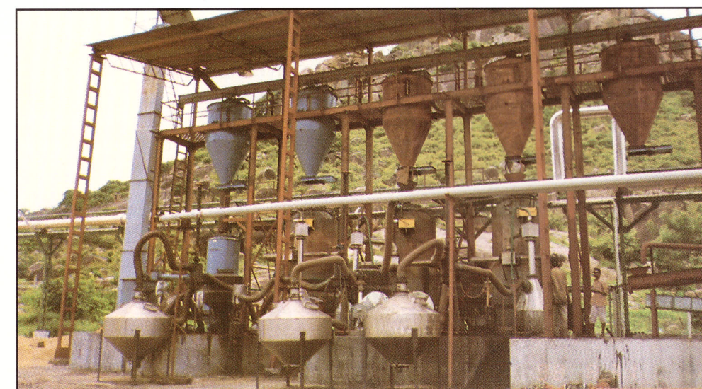
IREDA financed gasifier unit of 972 kW set up in village Raigir, District Nalgonda, Andhra Pradesh.
