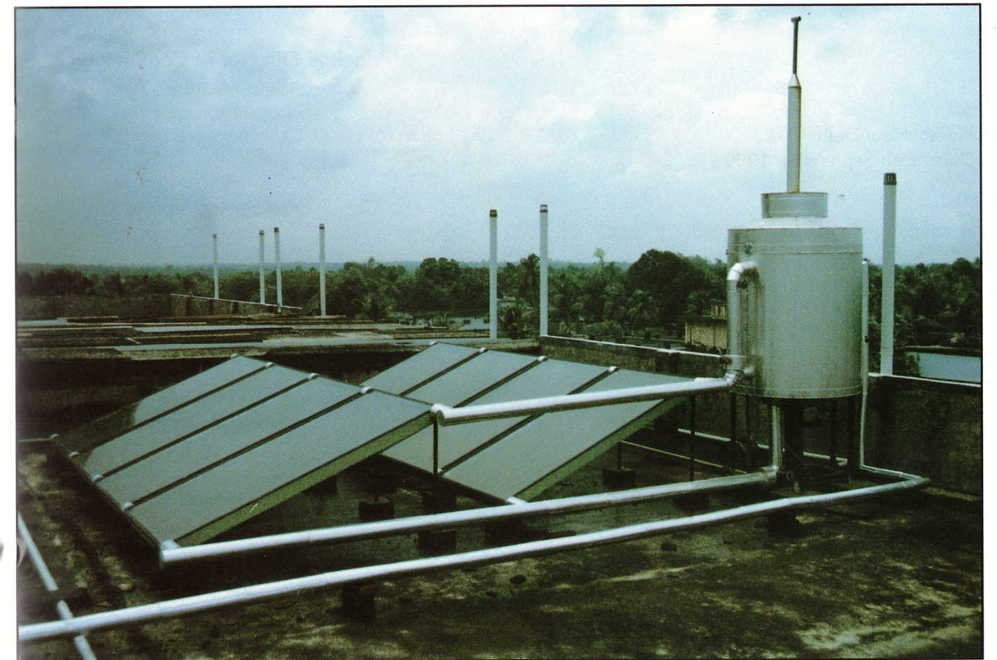
IREDA financed 3000 LPD Solar Hot Water System installed in a Hospital in Ernakulam District, Kerala.
