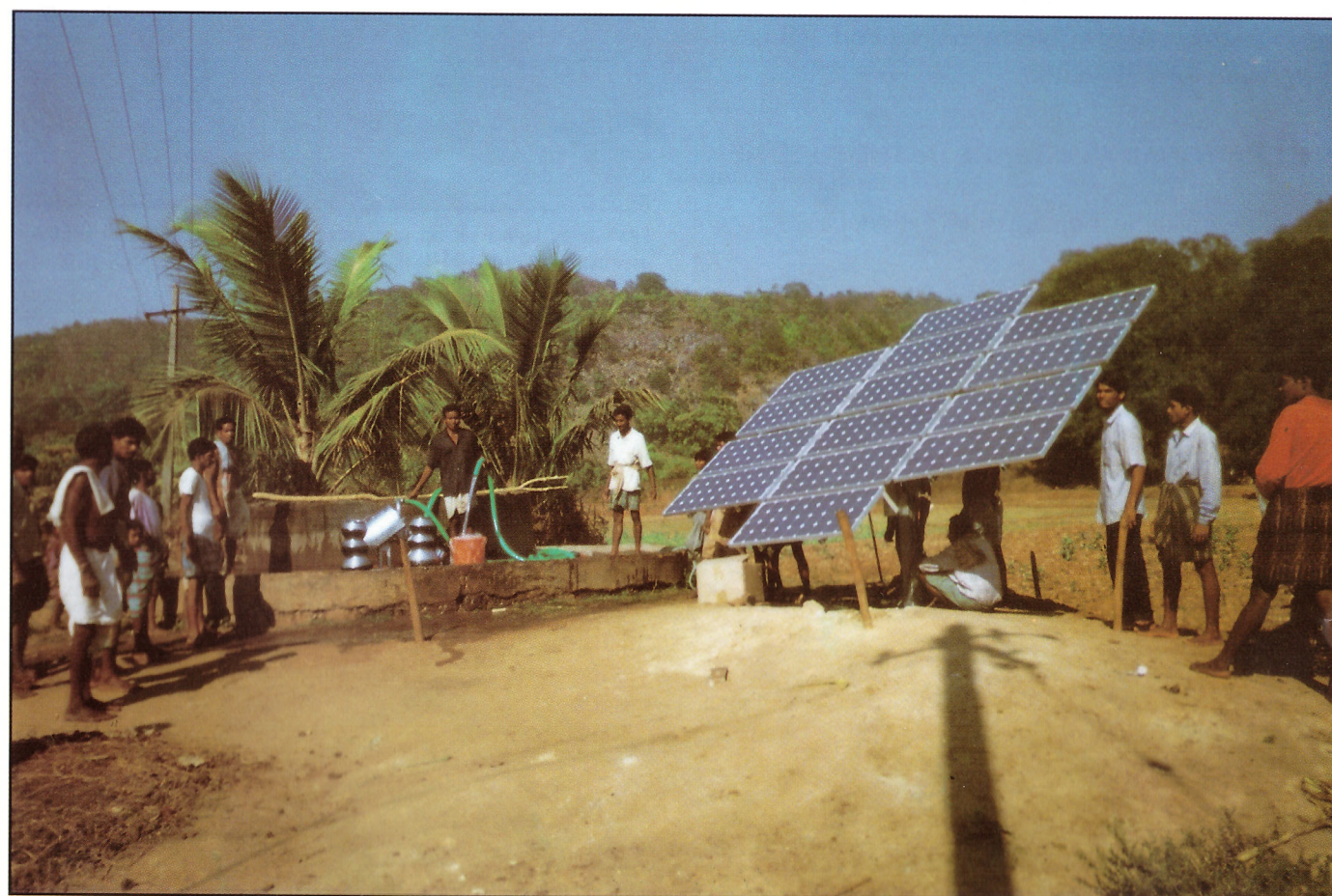
Solar Photovoltaic Water Pump installed under MNES Programme through IREDA in Village Gujji, District Srikakulam, Andhra Pradesh.
