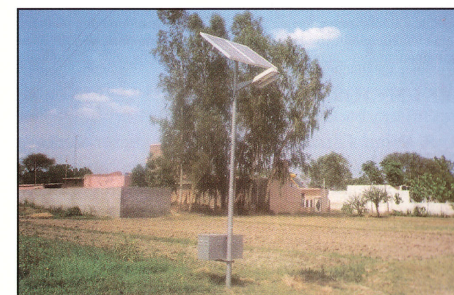
SPV Street Light installed under 'IREDA Akshya Urja Gram Scheme' in Village Bassi Kaso, Hoshiarpur, Punjab.
