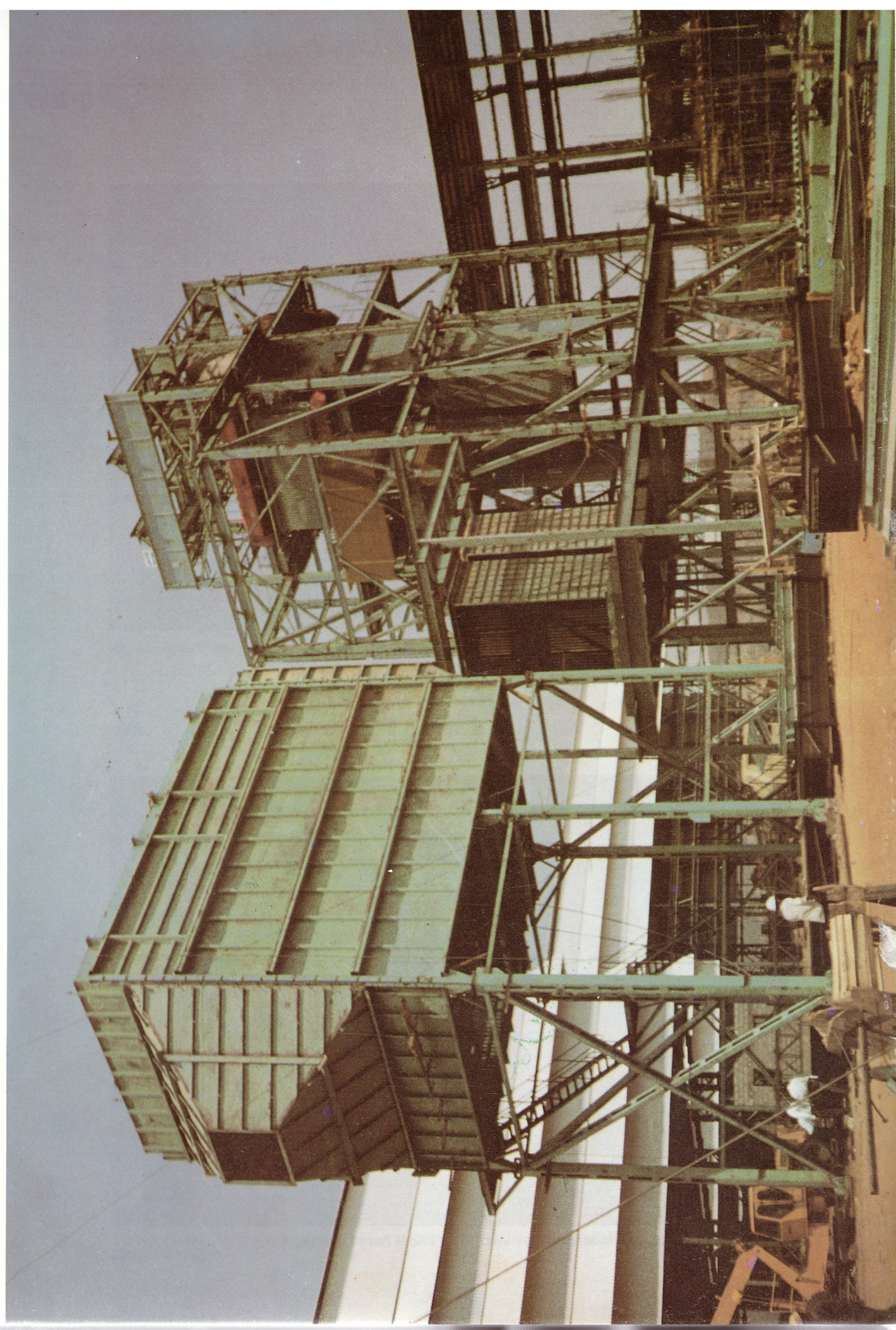
IREDA financed 22 MW Co-generation plant set up in village Duggavati, Bellary District, Karnataka, under ADB Line of Credit.
