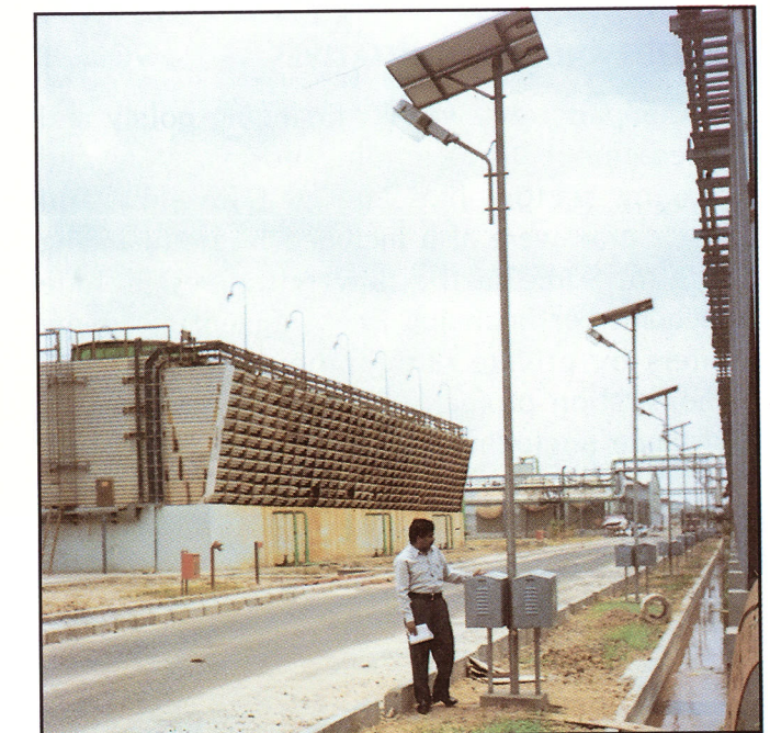
SPV Street Lights set up in a factory in Ahmedabad with IREDA's assistance under World Bank Programme.
