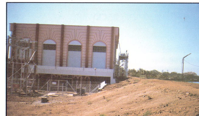
2.8 MW Mini Hydel Project set up at Gokak, Karnataka with IREDA's assistance, under World Bank Programme.
