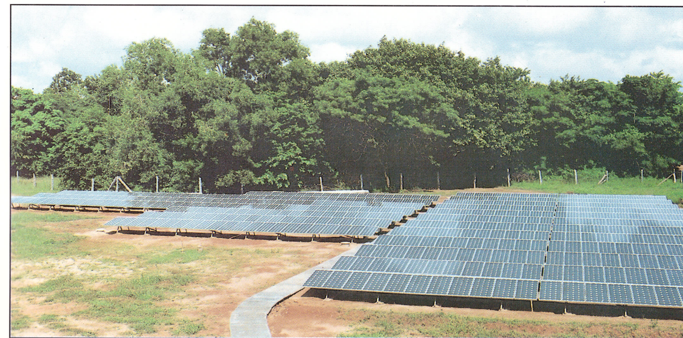
IREDA financed 36.2 KW SPV Power Plant at CSR, Auroville, Tamilnadu.
