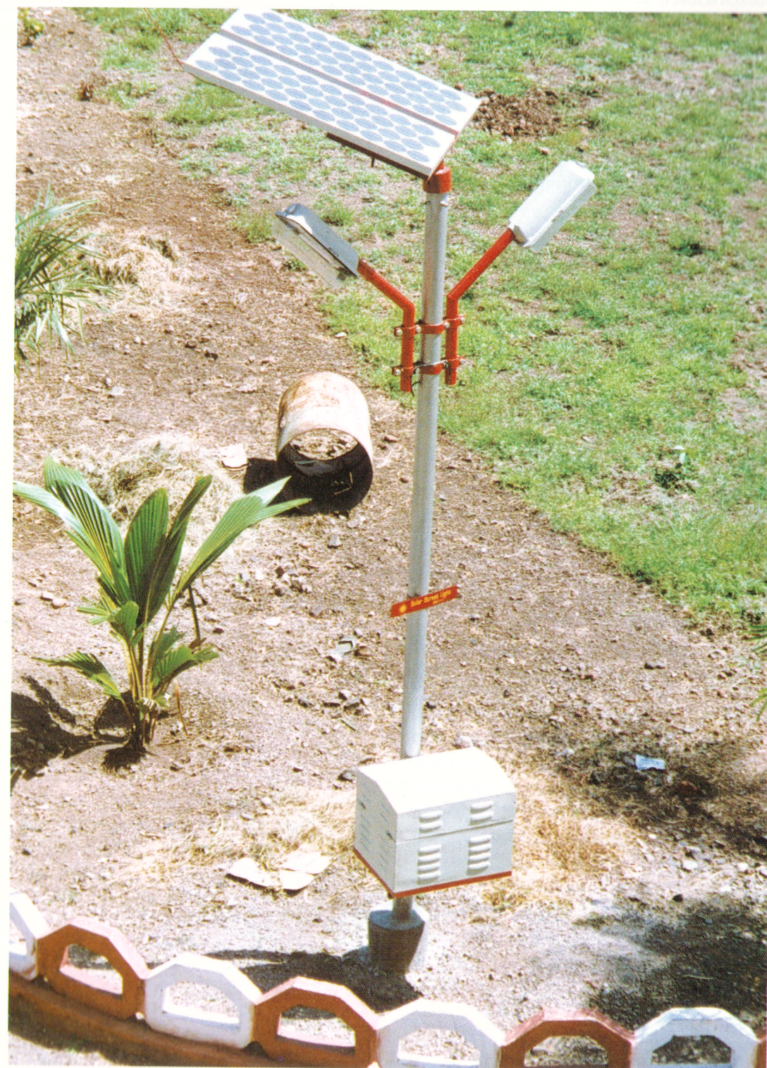
Solar Photovoltaic Street Lighting financed by IREDA, under the SPV Market Development Programme of World Bank, in Nasik district of Maharashtra.
