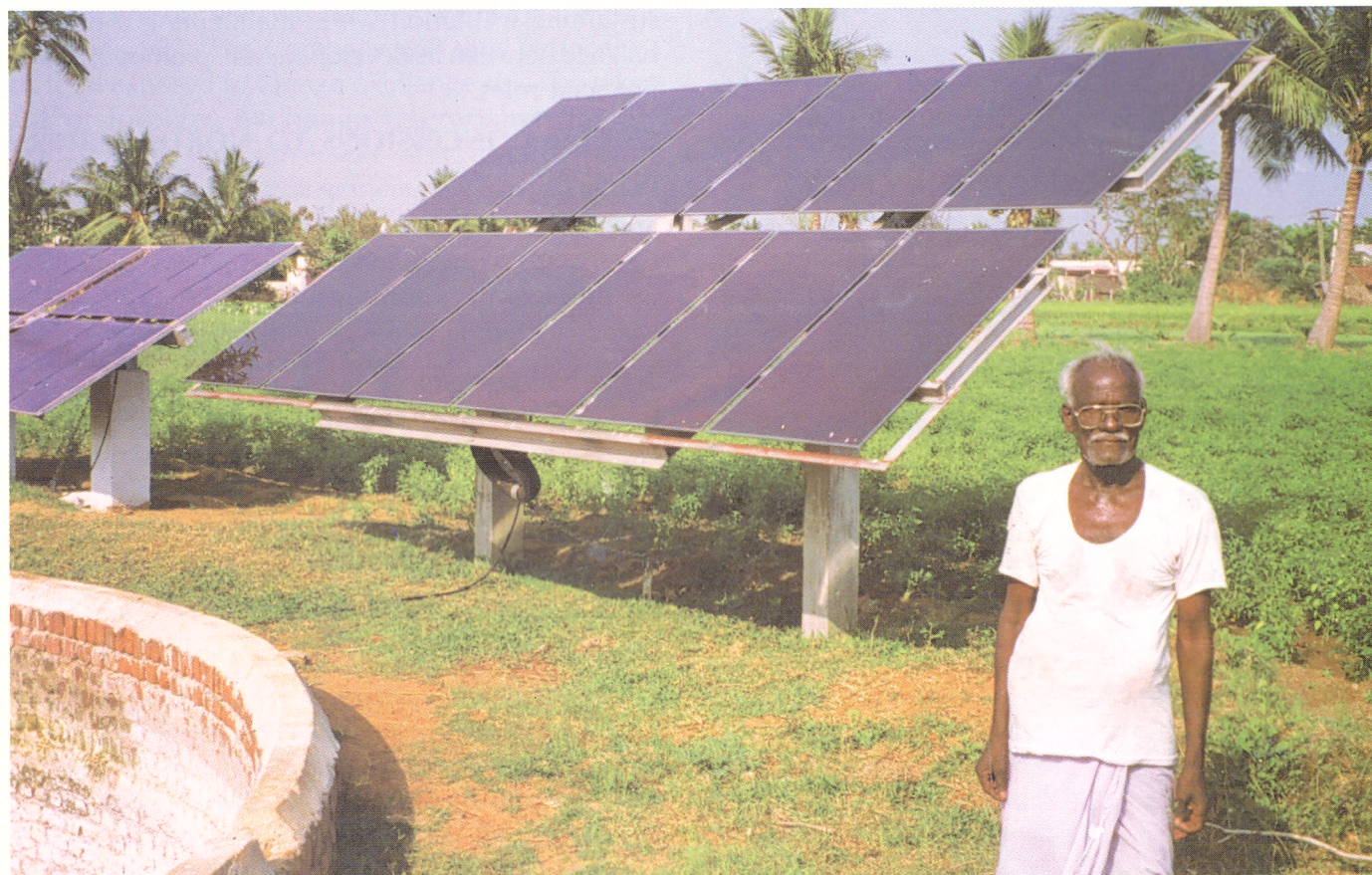
Solar Photovoltaic Water Pumping System for Agriculture, funded by IREDA under the "SPV Pumping Programme" of MNES in MGR district of Tamilnadu.
