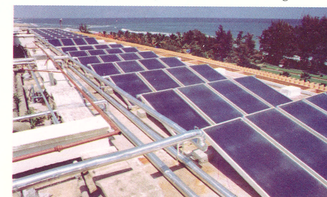
19000 LPD Solar Water Heating System in a hotel, installed with IREDA's assistance in MGR district of Tamilnadu.
