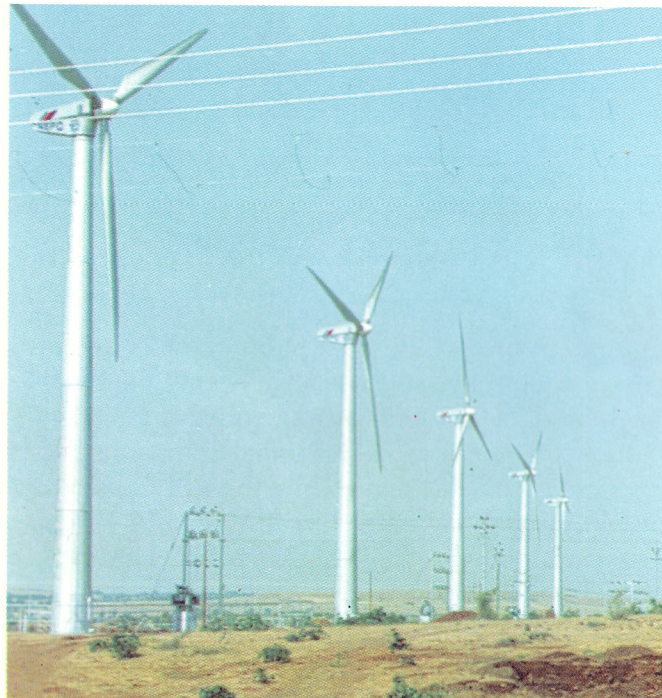
A Wind Farm in Madhya Pradesh set up by the MP Wind Farms Ltd., the Joint Sector Company of IREDA.
