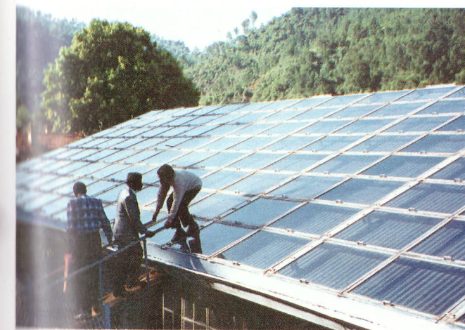
300 Sq. Mtr. Solar Air Heating System installed with IREDA's assistance in a tea estate at Conoor in Tamil Nadu.
