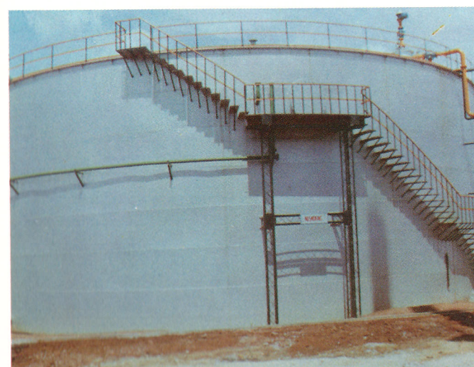
A view of 'Digester' of Biomethanation Plant set up with IREDA's assistance at Dharwar district of Karnataka
