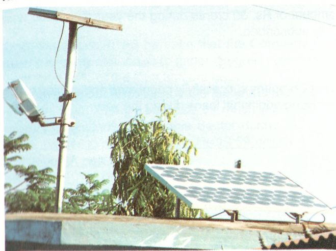
'SPV Street Lighting' financed by IREDA, under the 'SPV Market Development Programme' of World Bank in Coimbatore, Tamil Nadu.
