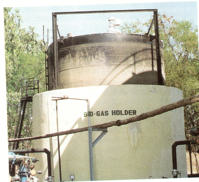
View of Biogas Holder plant alongwith gas pipe lines and Digester feed pipe line set up with IREDA's assistance at Sameerwadi Distt., Bijapur, Karnataka.
