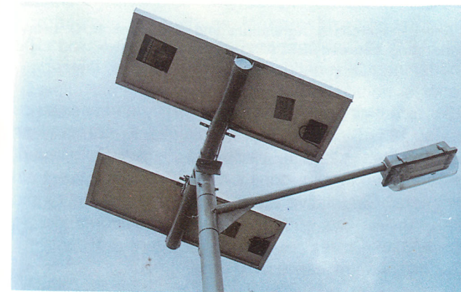
Street Lighting Systems with IREDA's assistance under SPV-MNES Programme in Gujarat.
