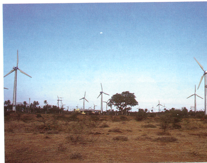
IREDA financed 0.75 MW Wind Farm Project in the State of Tamil Nadu
