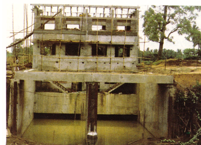
View of Power House from downstream side to upstream under a Small Hydro Scheme financed by IREDA in the State of Orissa.
