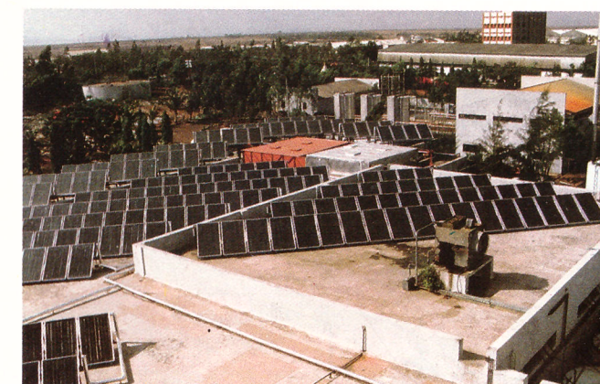
IREDA financed Solar Water Heating System of 50,000 LPD Capacity in Dist. Kolhapur, Maharashtra
